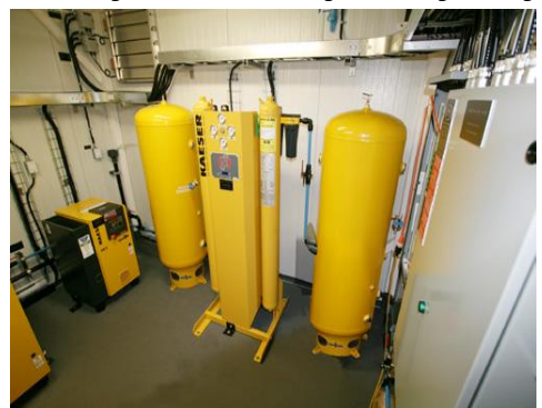
Dessicant oxygen driers and compressors
