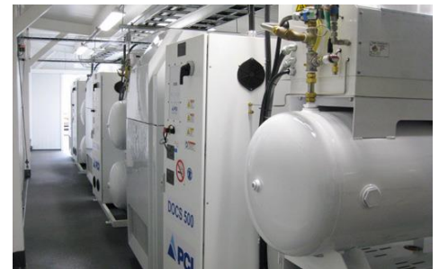
O 2 generators inside the gas handling building
