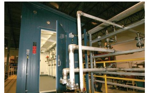
Liquid SO 2 tank above storage tank, Ontario
